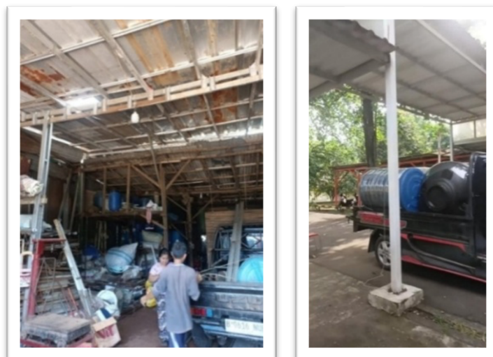
Fig. 6. Fabrication process of the lightweight steel frame and procurement of system components
