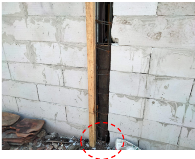
Fig. 13. Sloof is not tied to the foundation
