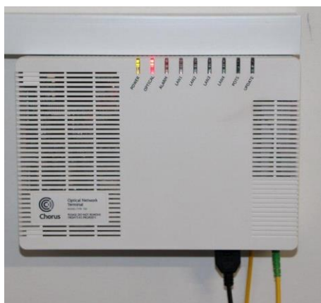
Gambar 5 ONT ( Optical Network Terminal )
